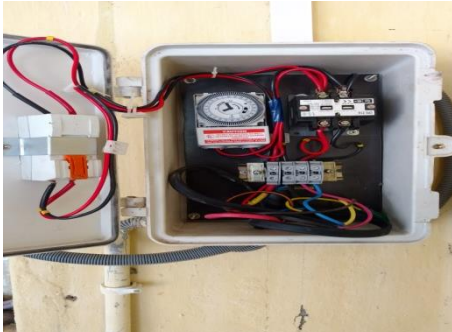
Provision of Occupancy sensors
