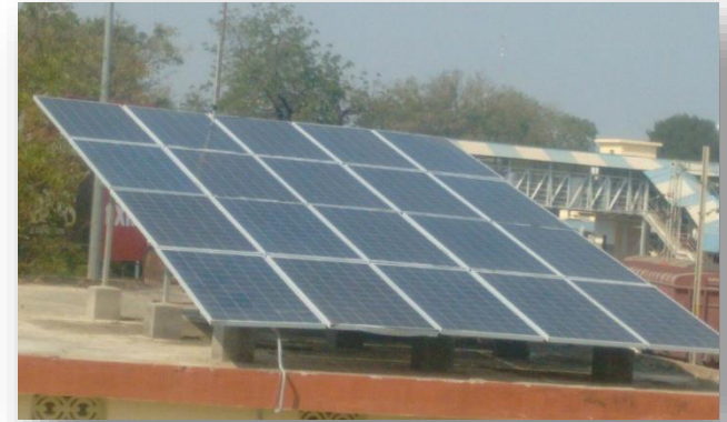
5 HP solar pump panels
