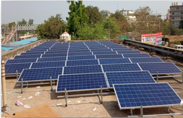
On site 100 kWp solar plant,
