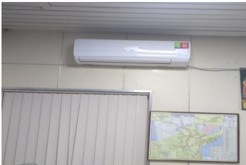
Energy efficient inverter type AC units
