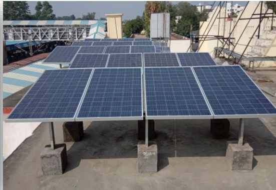
On site 10 kWp solar plant
